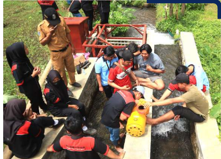
● The process of installing the waterwheel in one of the river streams
